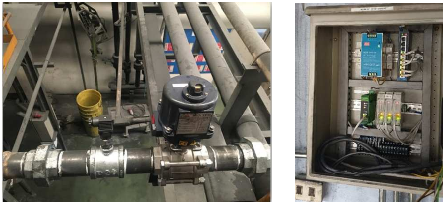
FIGURE 6. Examples of devices installed at the plant and connected in the cabinet
