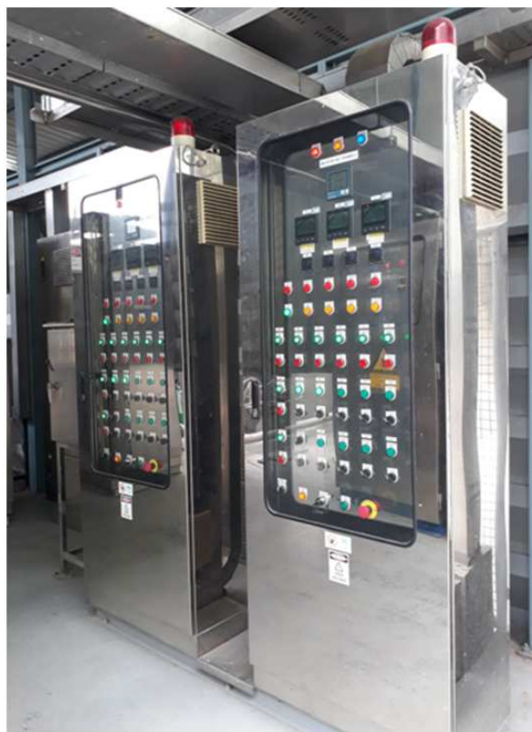
FIGURE 2. Control panels of two multi-stage wet scrubbers at field site
