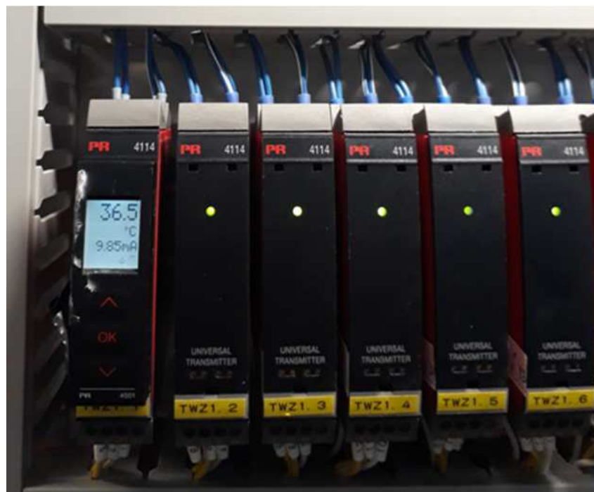
FIGURE 6. Display and programming module of the transmitter inside the power cabinet
