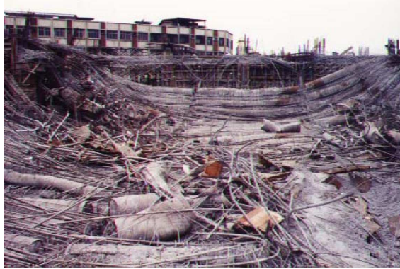
FIGURE 1. Fallen formwork used as scaffolds for constructing in Chin-Shi Elementary School in Taoyuan
