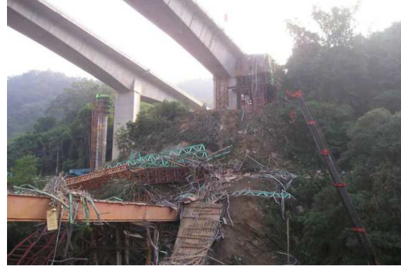
FIGURE 2. Fallen formwork used as scaffolds at the Beishan Interchange on Freeway No. 6 in Nantou County
