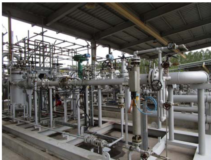
FIGURE 2. Flow metering skid for condensate residue custody transfer
